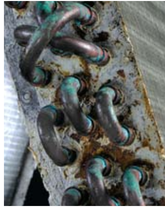
Copper tube and galvanized steel tube sheet after 500 hours in a controlled corrosive environment.
