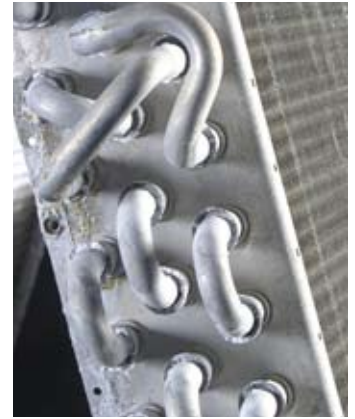
Aluminum tube and tube sheet after 500 hours in a controlled corrosive environment.
